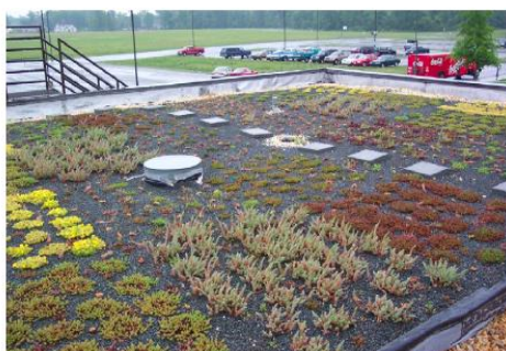
(a) Telhado verde do Wayne Community College, Carolina do Norte, EUA.
