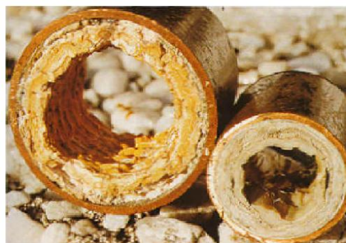
Fig. 1 Scale removed from a water pipe sectioned from a boiler
