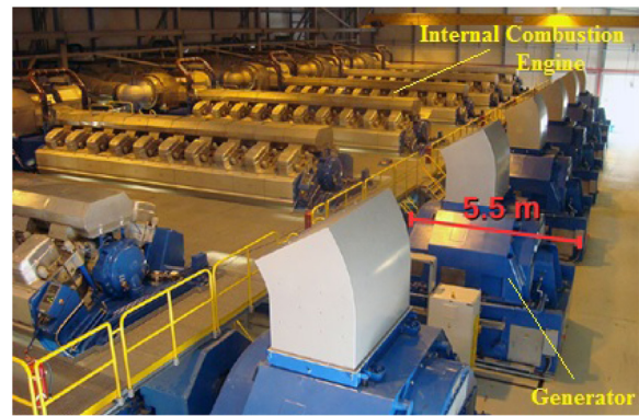
Fig. 20. In-service 28-MVA generation units in a hangar of Suape II Power Station [28].
