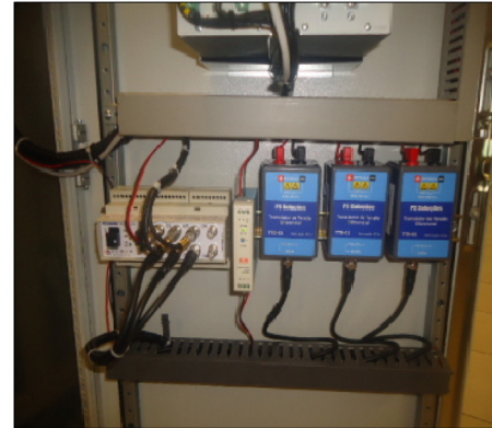
Fig. 19. Prototype installed at a Panel of Suape II Power Station.
